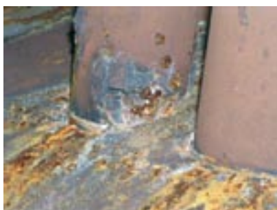
Corroded boiler furnace dome and convection tubes.
