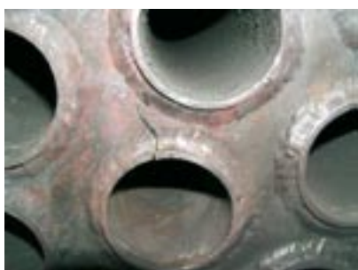
Creep cracks in a boiler end plate due to long-term overheating.
