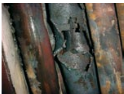
Tube burst due to short-term overheating.
