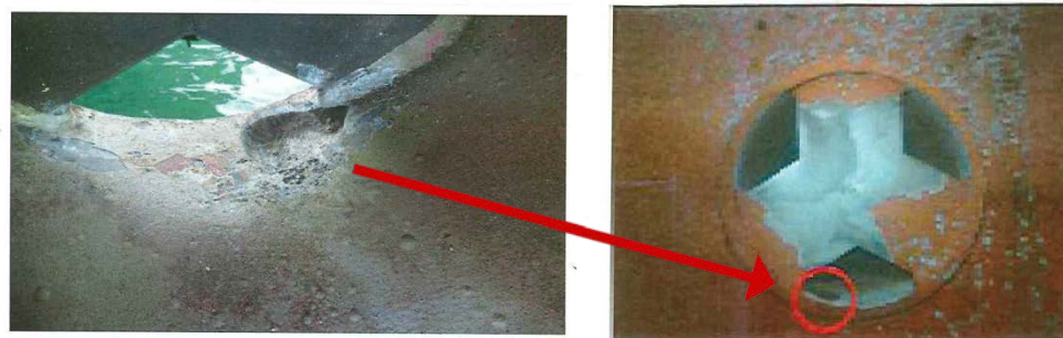
Picture 2 Corrosion around weld between distance piece and bluff body
