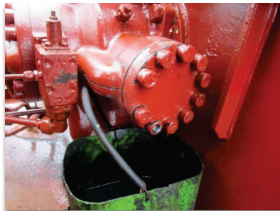
Photo 2: Ruptured motor housing to windlass experienced during attempted recovery of anchor
